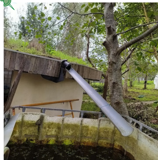
Green water treatment roof in Abrazo House
